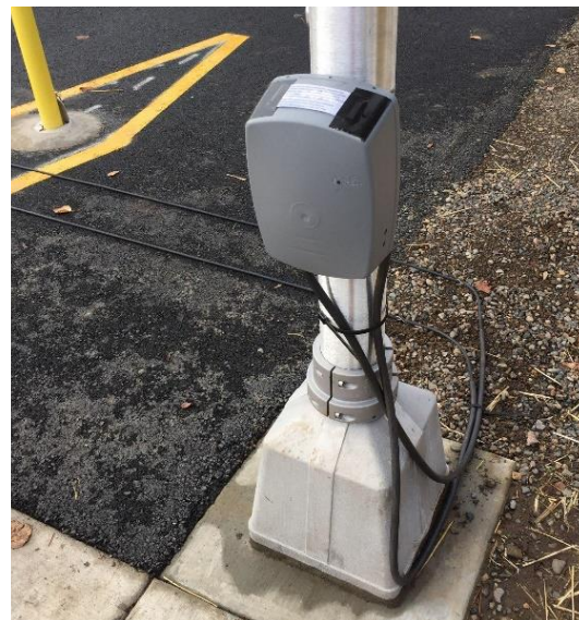
Figure 3: Pyro Box on Pole
