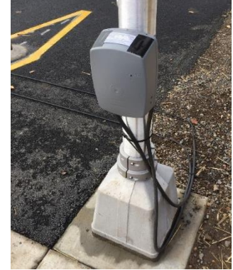
Figure 1: Count Equipment Installed in the Field
