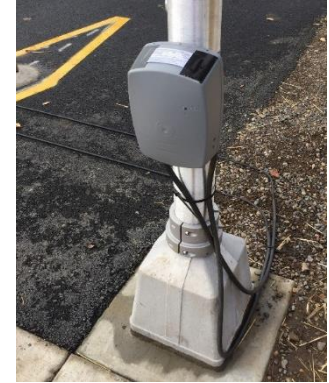
Figure 1: Count Equipment Installed in the Field
