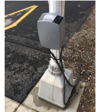
Figure 1: Count Equipment Installed in the Field
